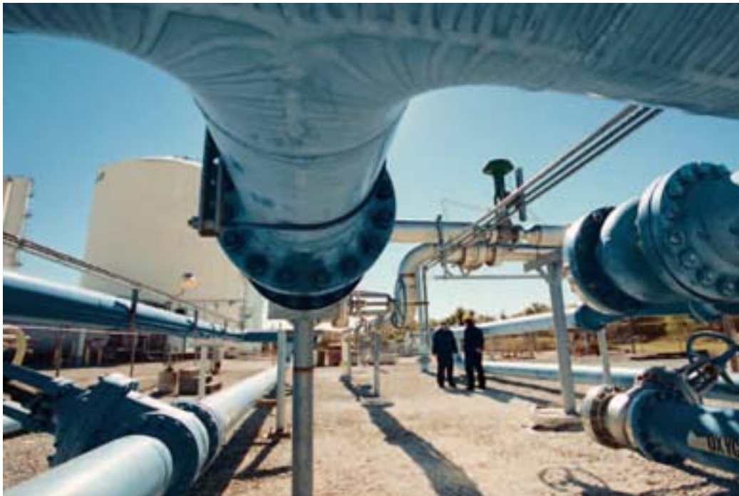
Figure 24. What a hydrogen pipeline might look like coming into a terminal or other gathering station (Photo downloaded from Praxair 2003 Annual Report, available at www.praxair.com )
