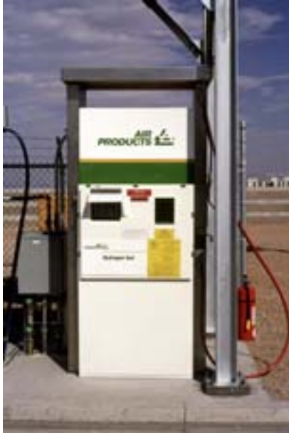
Figure 13. A picture of an actual hydrogen dispenser (photo obtained from Air Products website, at www.airproducts.com ).
